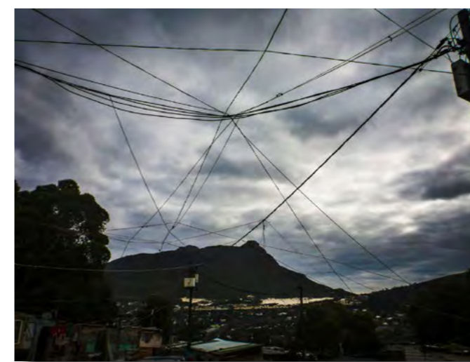
Figure 5.23: The overhanging wires present numerous challenges for emergency vehicles
