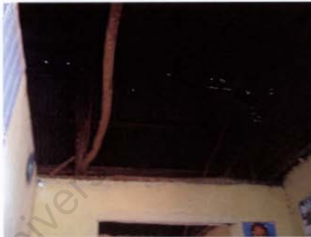
Figure 111: None of the houses had ceilings installed. By installing ceilings, more light could be refracted and used within the desired area.
