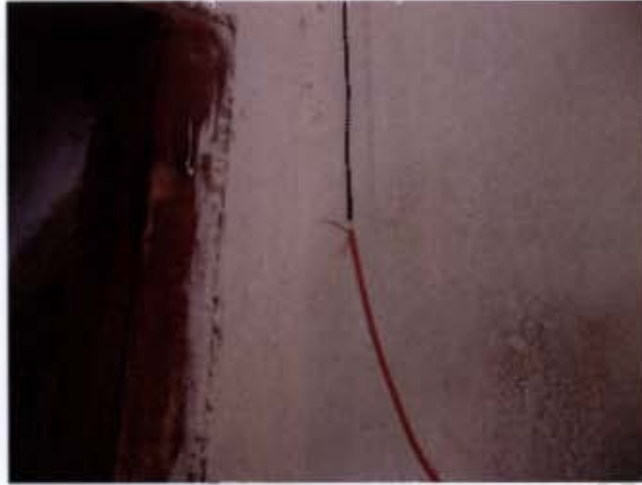
Figure 112: A contact to switch on and of the white LEDs in a room. Such weaknesses in the system installation reduced the sustainability of the project.
