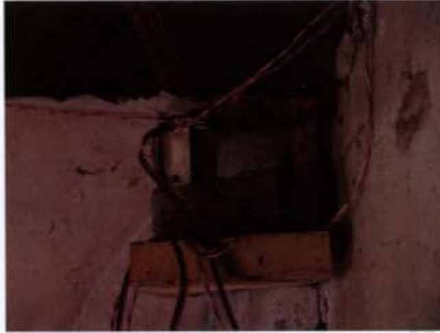
Figure 110: The battery used to store charge from a solar PV system
