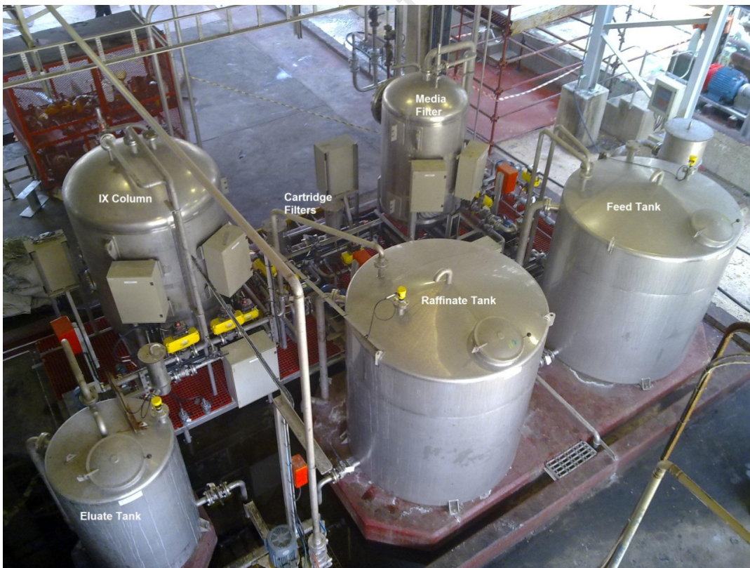
Figure 6-1: Zinc ion-exchange plant at RBMR.
