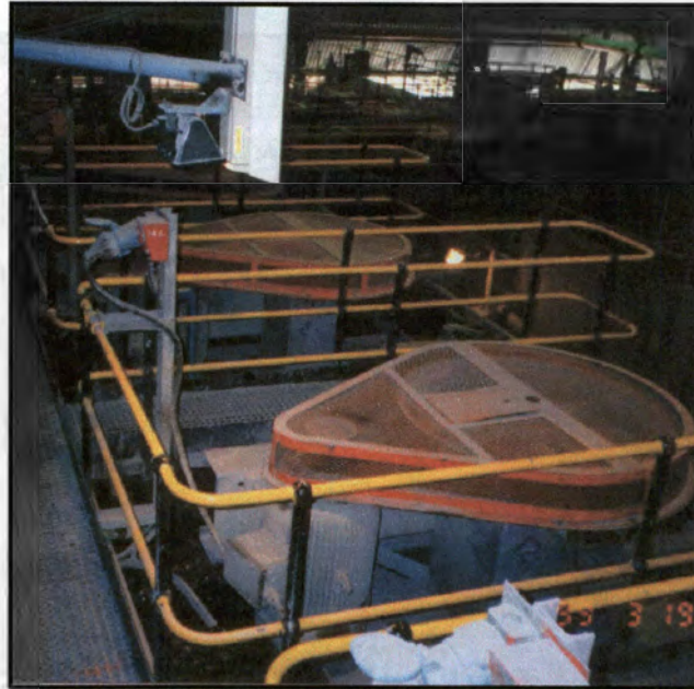
Figure 3.13: Camera assembly and spotlight mounted above one of the rougher cells on the Amandelbult Primary Rougher bank.
