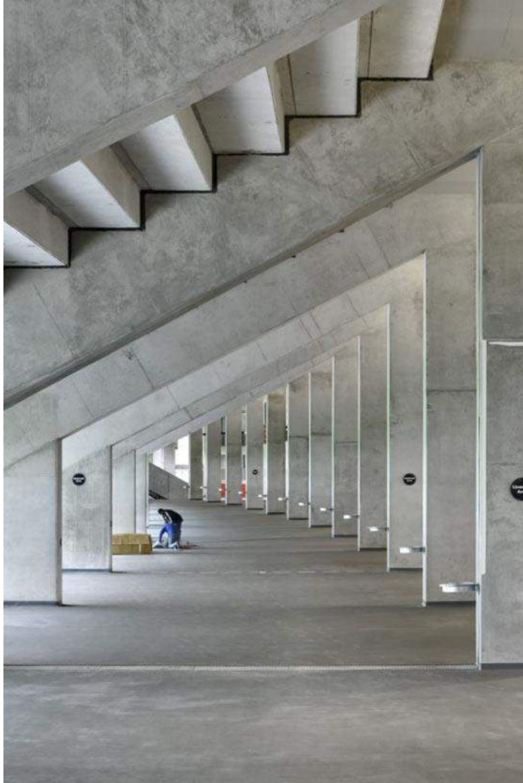
Figure 24 The Stadium has a robust concrete structural expression as seen in this image from the Level 2 concourse under the middle tier of seating
