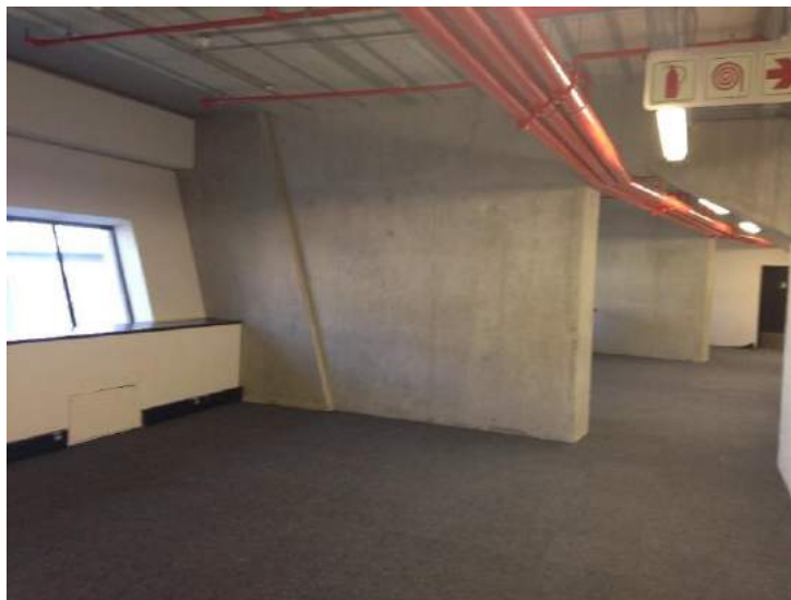
Figure 27 Photograph of an empty office on Level 4 with openings on one side and a passage to the right
