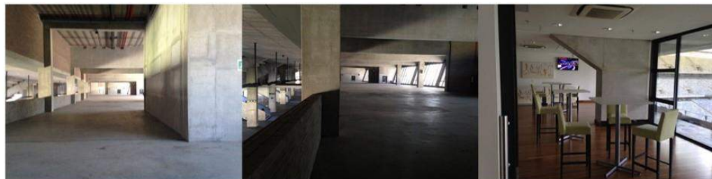
Level 3 has a generous double volume and overlooks the concourse below. Level 4 is obscured from it by a brick wall
