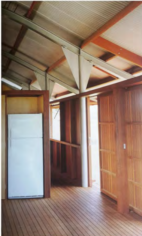
Figure 49: This image clearly shows the two main materials which constitute the hybrid structure of the Marika-Alderton house. The hardwood structural components span the length of the house, while a structural steel frame achieves stability across the width.
