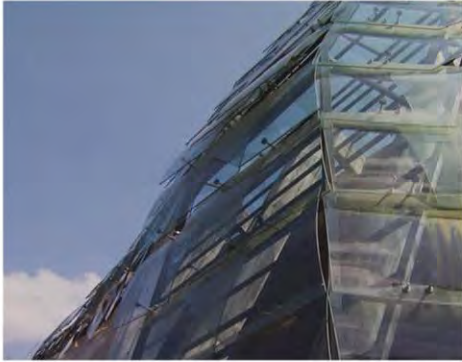
Figure 47: Reclaimed car windows provided an economically efficient option for constructing the glass portion of the building
