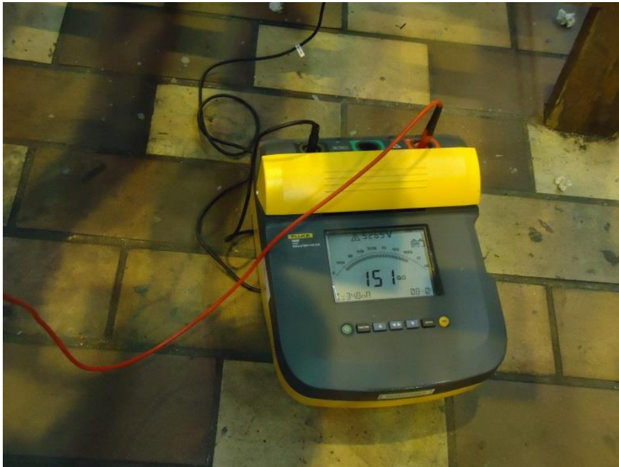
Figure 4-1: Megger, used for measuring IR and PI
