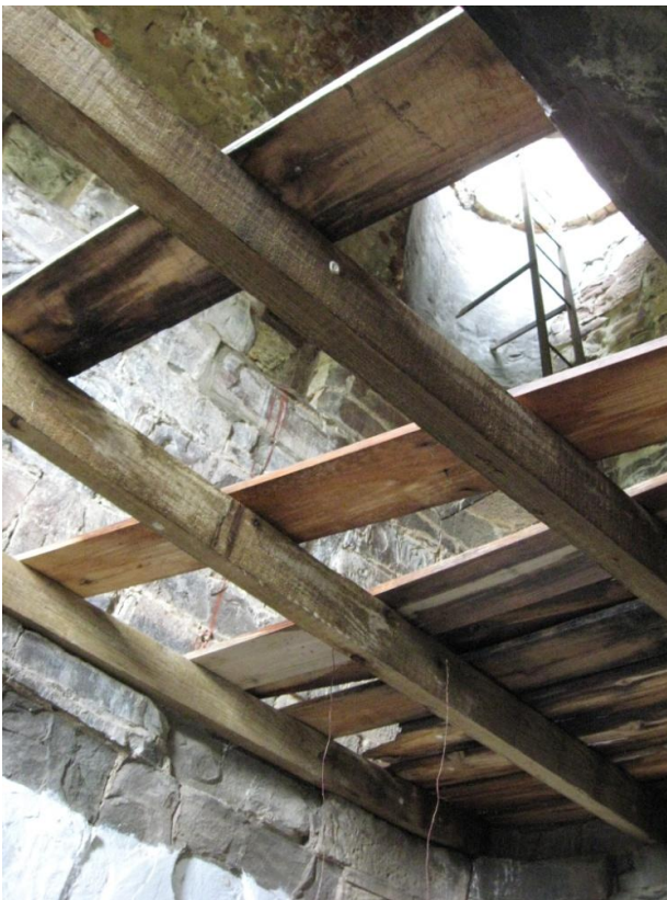
Figure 24 View from inside the tower of the ladder leading to the roof on which the gun was mounted, 2011 (Photograph: S I Blackbeard)
