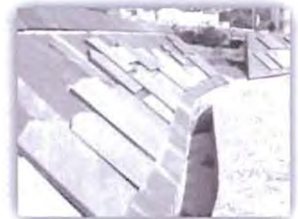
Figure 12b – the 'wave wall' relating to its seaside context: Garden of Remembrance, Uytendogaardt (Thalassinos, 2008)
