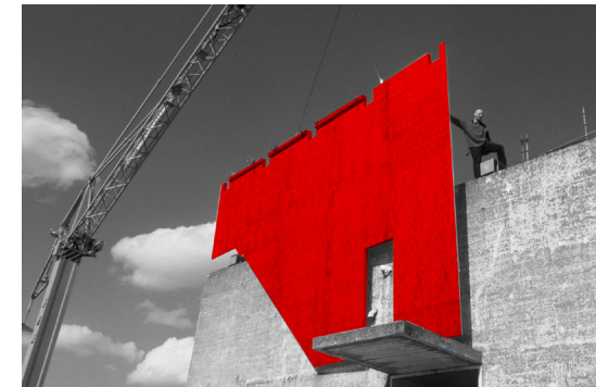
Figure 41: The parasite is constructed directly onto its host by lifting the prefabricated elements with a crane.
