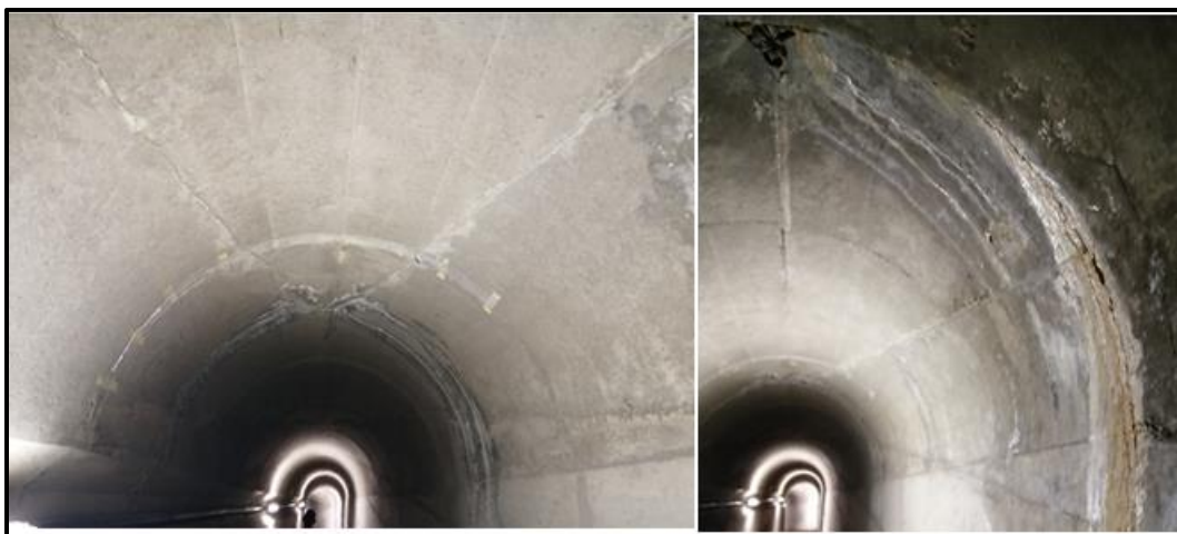
Figure 28: Cracks within the Oanob Dam Gallery
