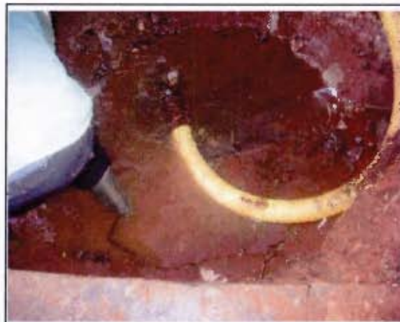
Figure 5.8: Leakages in the water supply system, Maputo (FIPAG, 2007)
