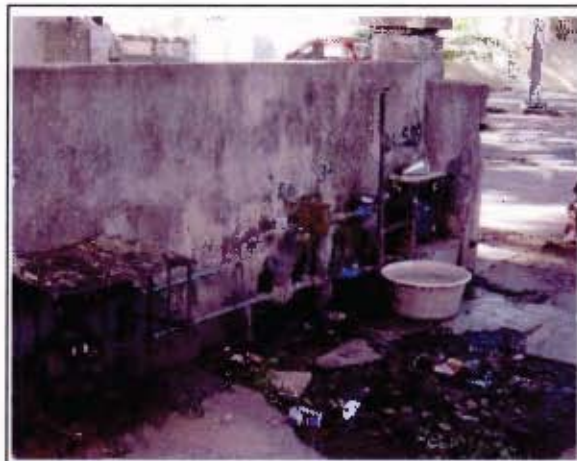
Figure 5.7: Leakages and faulty meters at consumer's side, Maputo (FIPAG, 2007)
