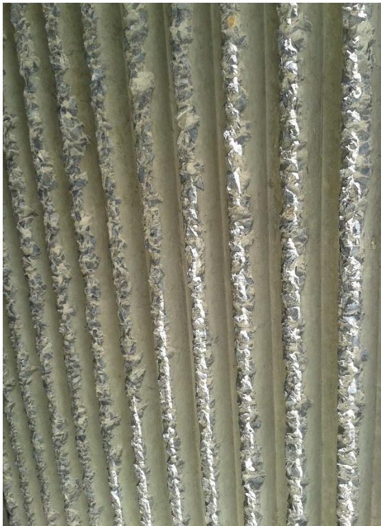
Figure 31: Close-up view of repaired stipple detail on 27 Wale Street. Image taken on 09-11-2016.
