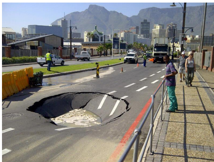
Figure 20: Damage to structures due to formation of sinkholes on dolomitic soils (Savage, 2014).
