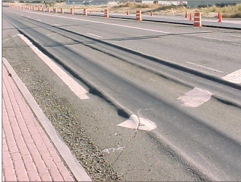
Figure 33: Rutting in paved road (sourced from Pavement Interactive)
