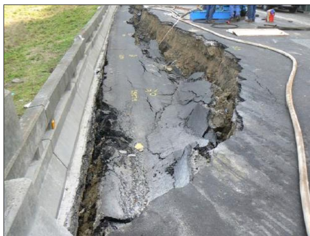
Figure 7: Stability failure of a pavement structure (SAPEM, 2013b).
