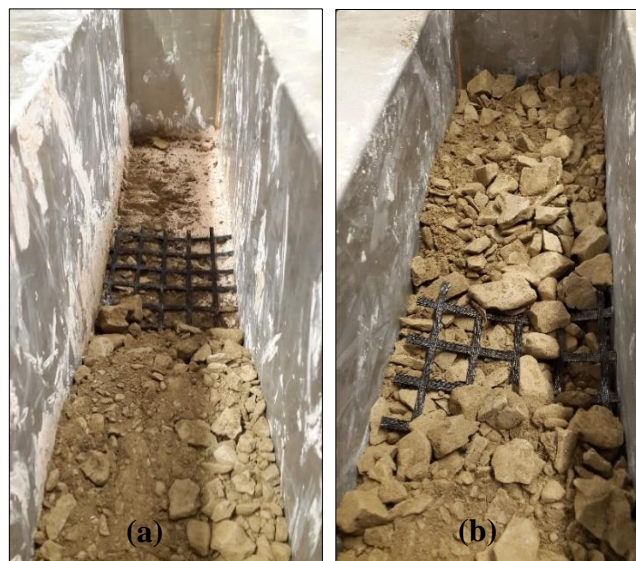
Figure 79: Geosynthetic layer placed (a) at the soil interface and (b) within the granular material layer.
