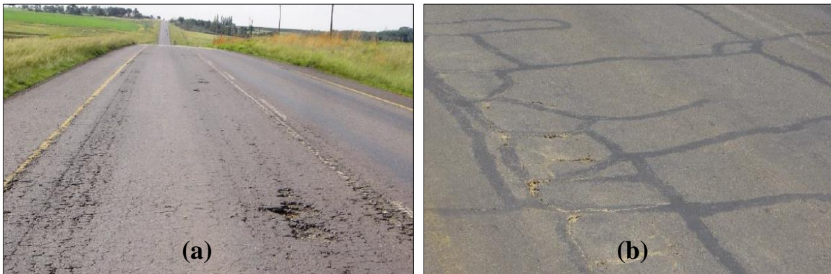
Figure 6: (a) Surface cracking and potholing and (b) Pumping of stabilized base and patching (SAPEM, 2013a)
