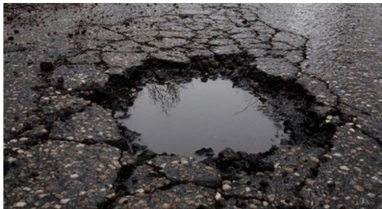
Figure 2.2: Poor Road infrastructure
