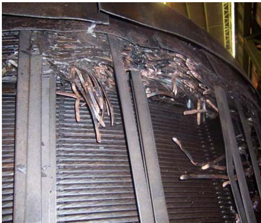
Figure 6-41: Damage to HV Winding
