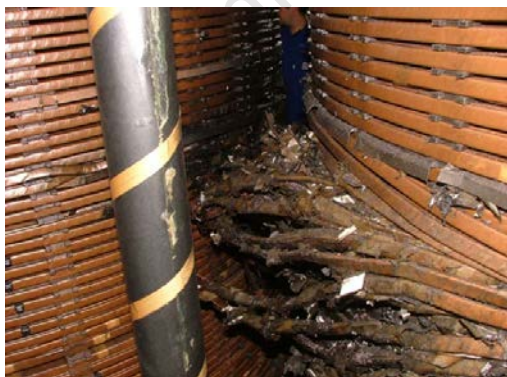
Figure 6-14: Case Study D - Damage on C phase HV winding
