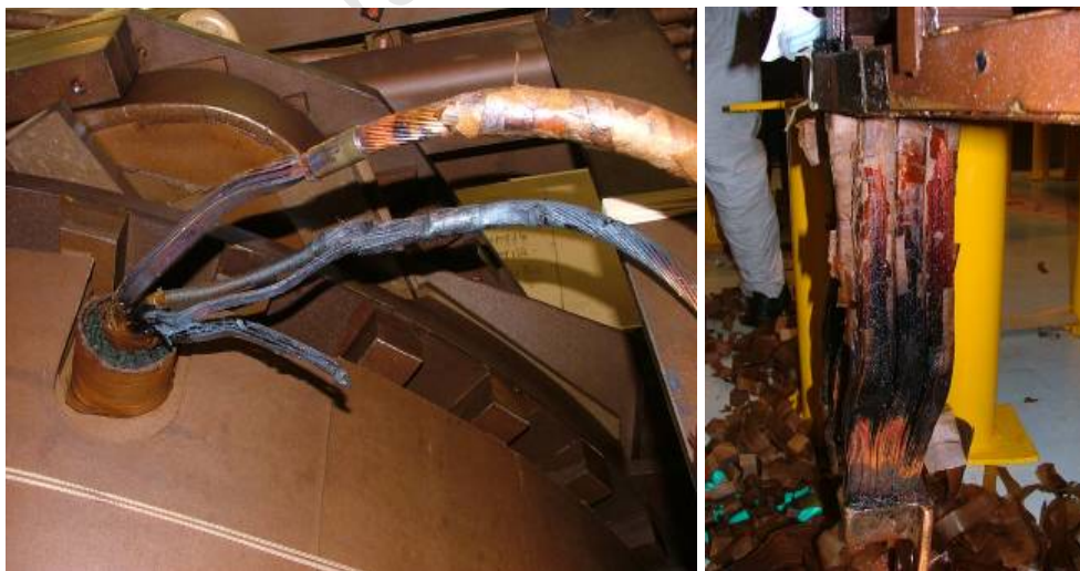
Figure 6-23: Evidence of Failure
