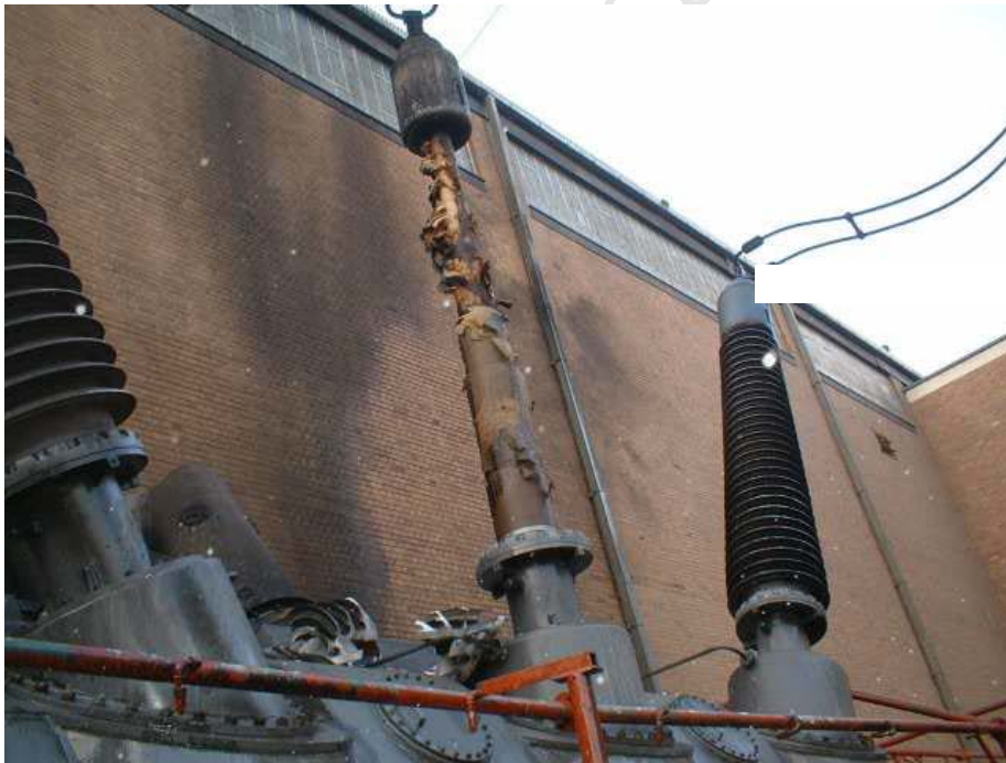
Figure 6-33: Damage B phase HV Bushing
