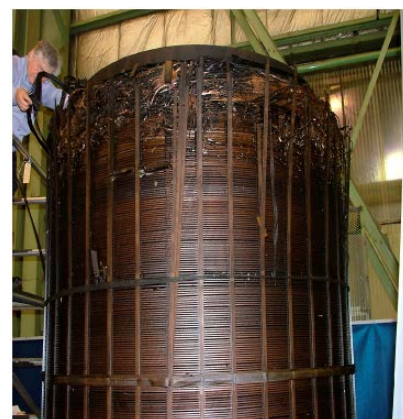
Figure 6-5: Damage on Top HV C Phase
