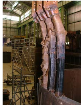
Figure 6-10: Thermal Heating LV Exit Leads
