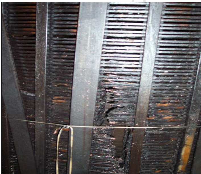
Figure 6-45: Damage C Phase LV Winding
