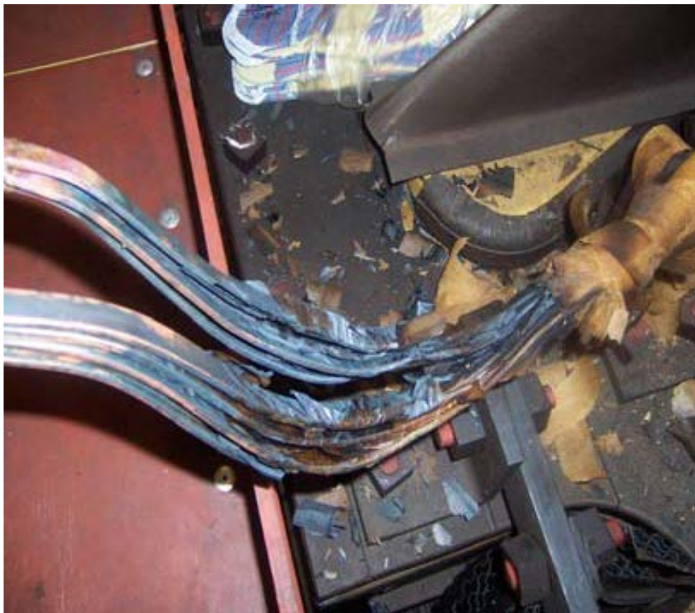
Figure 6-37: Damage to HV Leads
