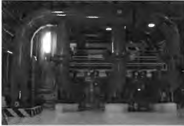
Figure 7.4: Industrial Plant Scene 2
