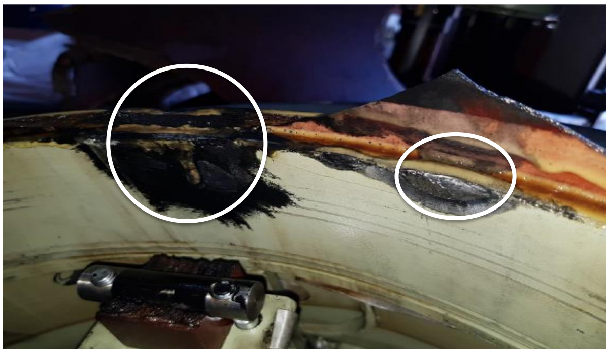
Figure 4-62: Damaged tap changer barrel
