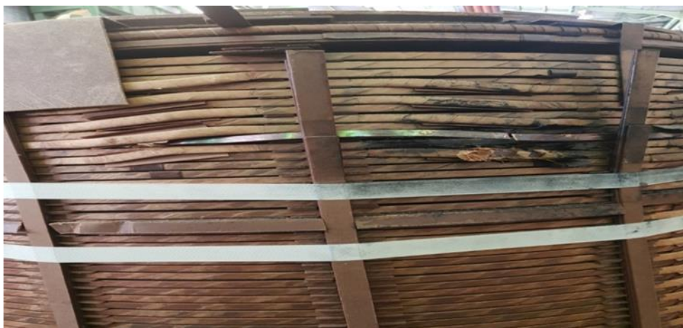
Figure 4-47: Faulted HV Winding
