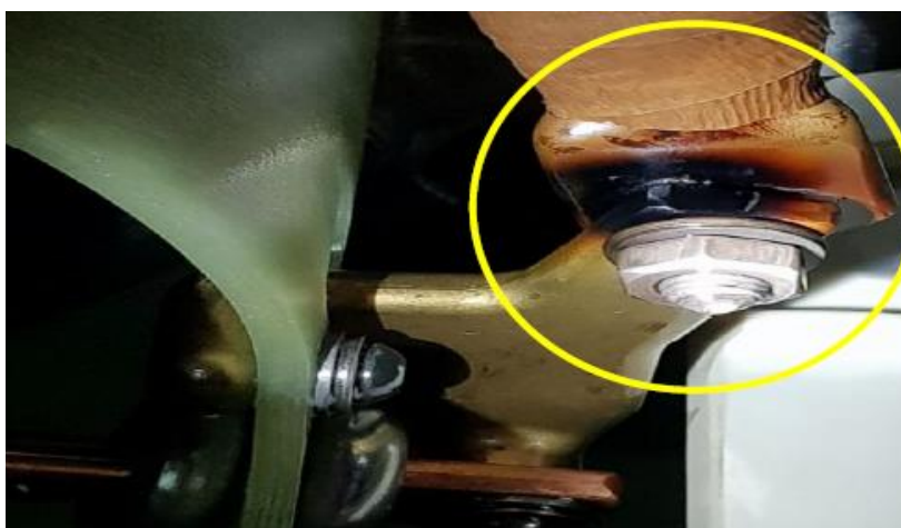
Figure 4-25: Overheating on changeover connection
