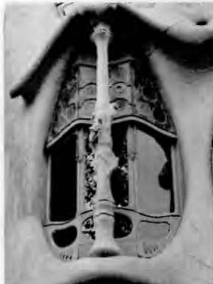
Figure 46: A close-up of one of the stone-framed window opening on the front façade.
