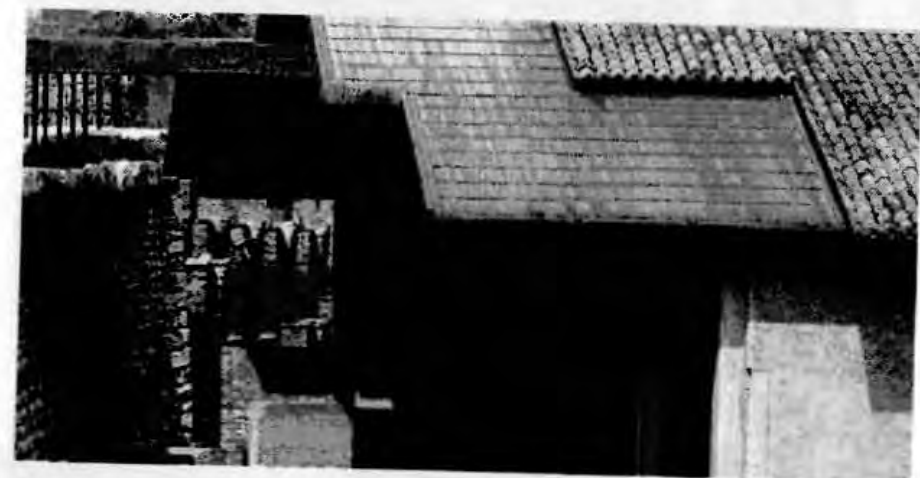
Figure 16: The roof over the Cangrande space: old and new is clearly distinguished from one another.
