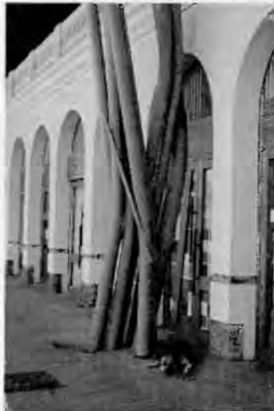
Figure 32. The twisted, tree-branch metalwork that supports the vault structure of the new roof.
