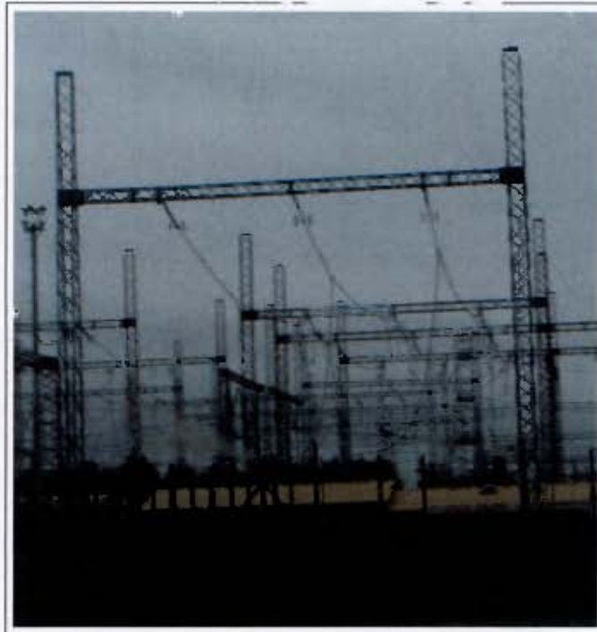
Figure 2.6. Powerlines in suburban area
