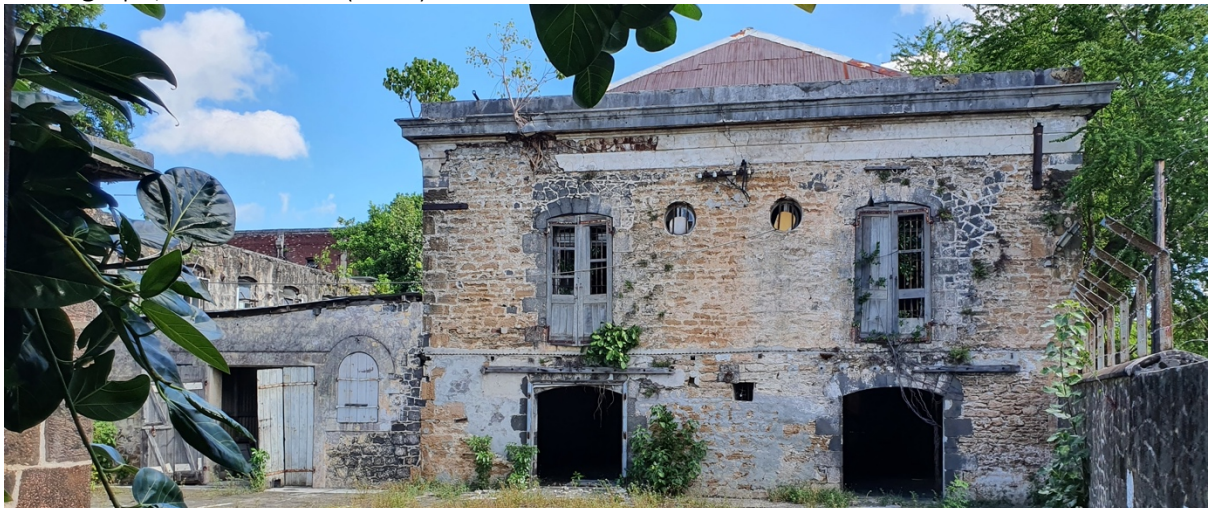
Figure 22: The grain store wing in a precarious state of repair. The local cut coral stone walls and tropical hardwood accessories are evident. The plastered French neo-classical cornice detail is also clear in this image. Photo by Author
