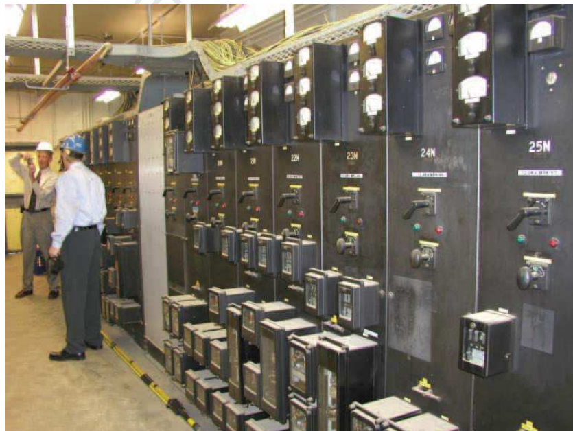
Figure 1.1 Phase-I relay with components that lack computing, memory, or communications capabilities required for substation automation [1]
