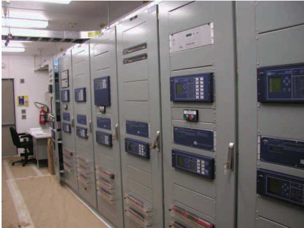
Figure 1.2 Phase-IV relays also called IEDs are used for Substation Automation [1]
