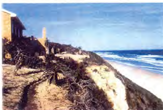
Collapse of steep slope immediately in front of holiday home under construction at "Blue Horizon", Eastern Cape
