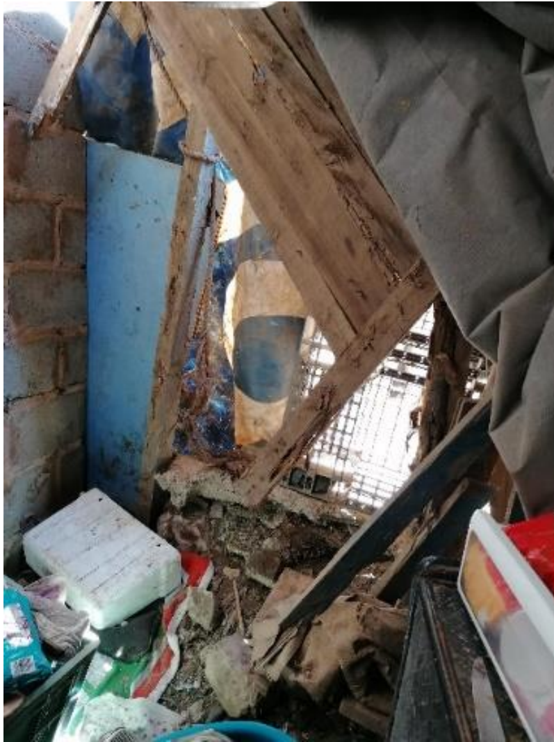
Figure 32. Damage to Mr. X's home after the floods
