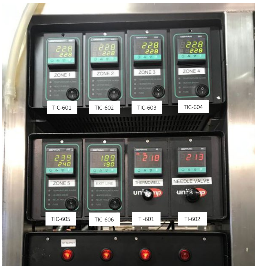
Figure A-11: Six Gefran 600 temperature-controllers for the 5-zone furnace (TIC-601, TIC-602, TIC-603, TIC-604, TIC-605) and first heating loop of reactor effluent line (TIC-606); two Gefran 40 temperature-indicators for the thermocouple placed inside the central thermowell (TI-601) and the other thermocouple positioned on the heated needle valve V-602 (TI-602)
