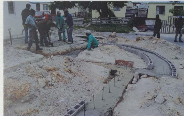
Thurs 30.10.2003 Left for work at 7:15 today Spent the day building the curved wall foundation and marking the places for the angle irons. The day went smoothly but slow. Three of Zukisa's friends are now helping out.
