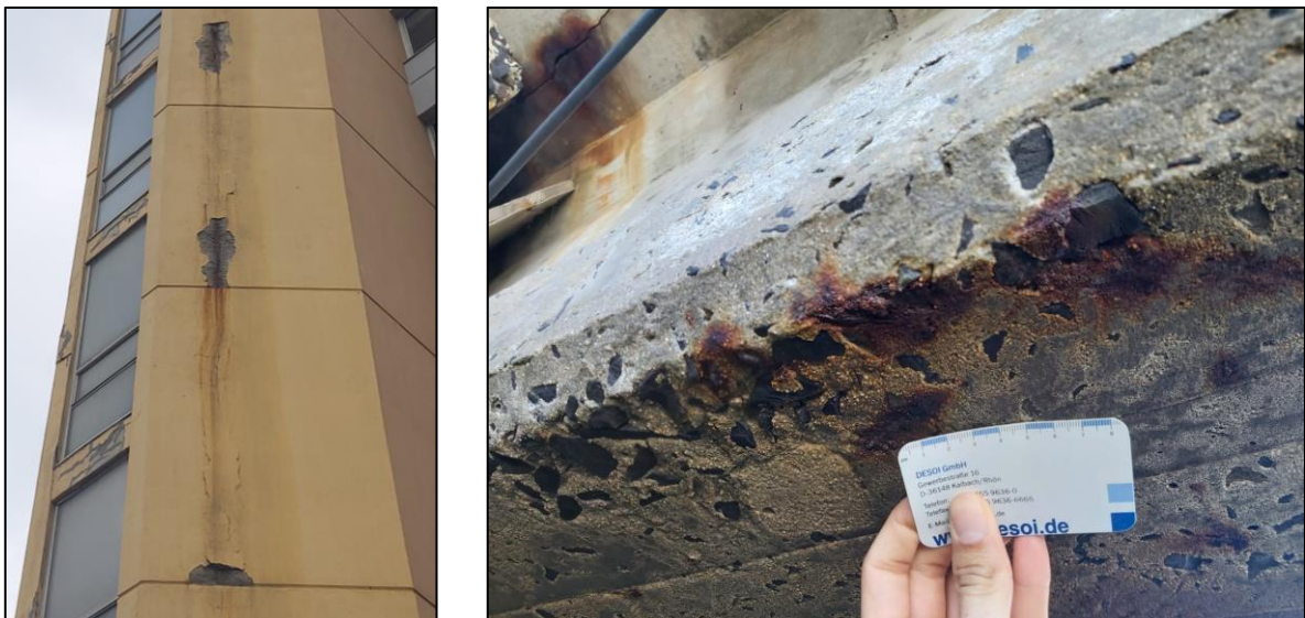
Figure 10 Effects of corrosion at TNPA House building (left) and Eastern Mole Approach Bridge (right)
