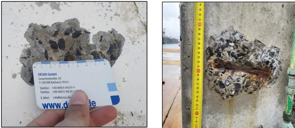
Figure 11 Pop-outs at the Quay 700 Prefabricated Substation (Left) and the Eastern Mole Pumproom (right)
