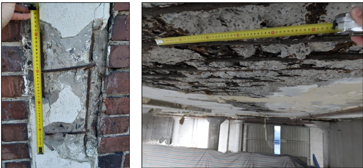
Figure 12 Spalling at the Unitie building exterior wall (left) and the B-Berth Shed (right)
