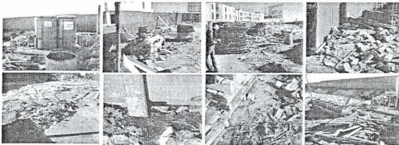
All damages to fencing, shade netting, footing and sandbags to be replaced. All construction related materials to be removed. Also all litter and food packaging to be collected and removed from Precinct 2.2
