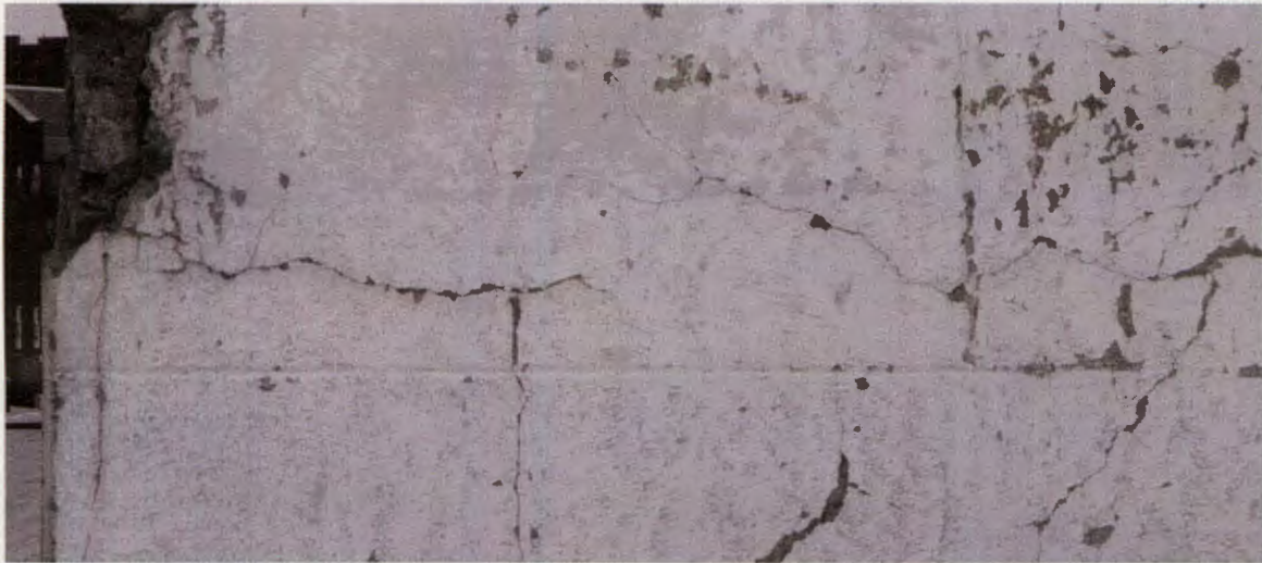
Fig. 61 Biodeterioration. Author's picture.
