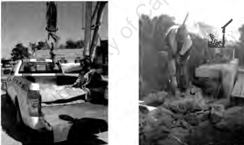
Figure 6.6: (Left) RCA-45 sample being collected from Concrete Units and being broken down by manual jack hammering before processing (Right)
