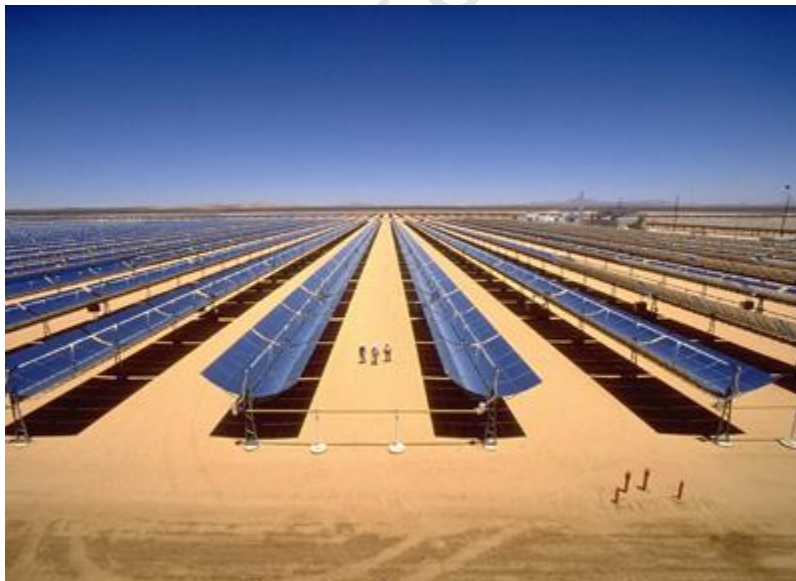
Figure 3-2 Typical parabolic-trough solar field
