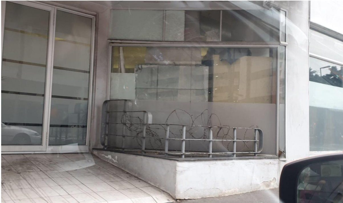
Photograph 3 Broken window syndrome - Neglect.
