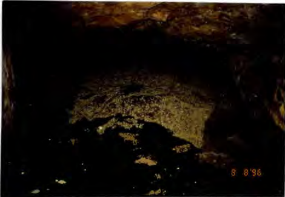
Figure 4.8. Photograph of main shaft water, with precipitate covering the surface.
