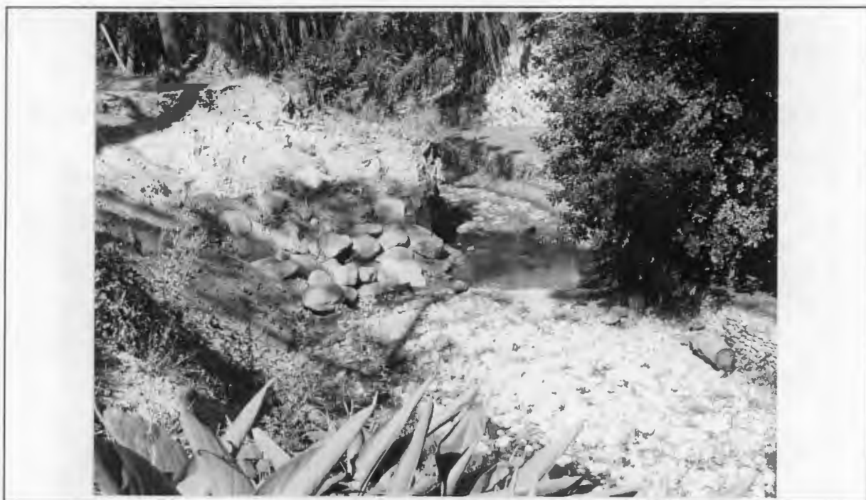
Figure 8.11: The same bank after regrading, showing the establishment of indigenous vegetation and the placing of boulders
