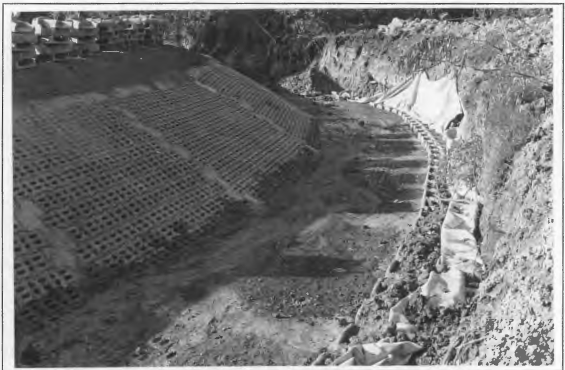
Figure 7.7: "Armorflex" interlocking blocks being used to stabilise a the bed and banks of a channel
