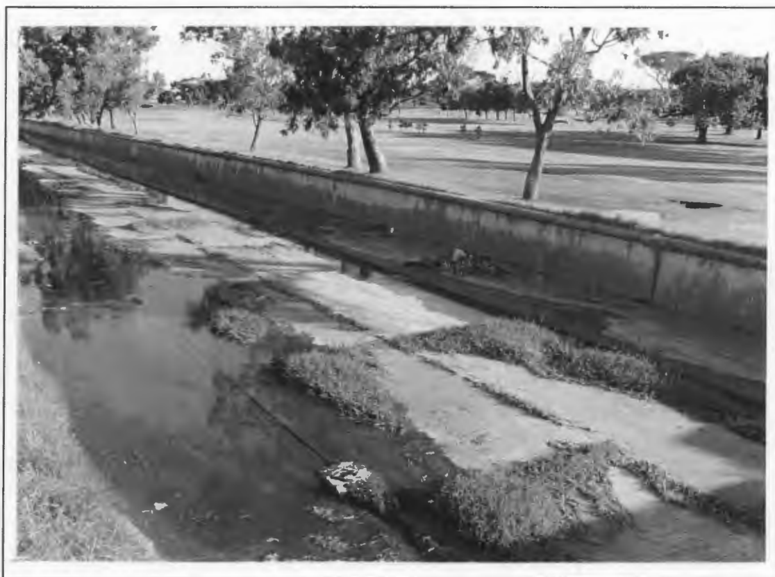
Figure 8.4: A typical section of concrete-lined channel in the lower reaches of the Liesbeek
