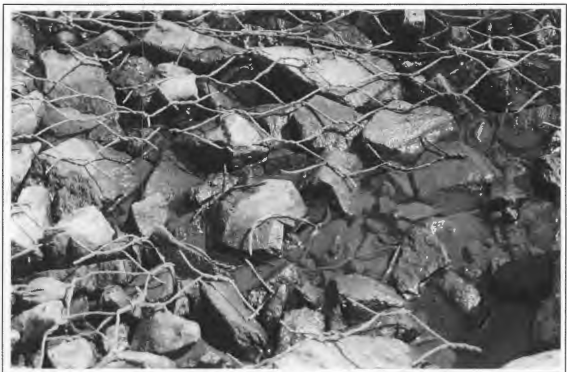
Figure 7.14: Once damaged, gabions lose their effectiveness and can become a hazard to people and animals
