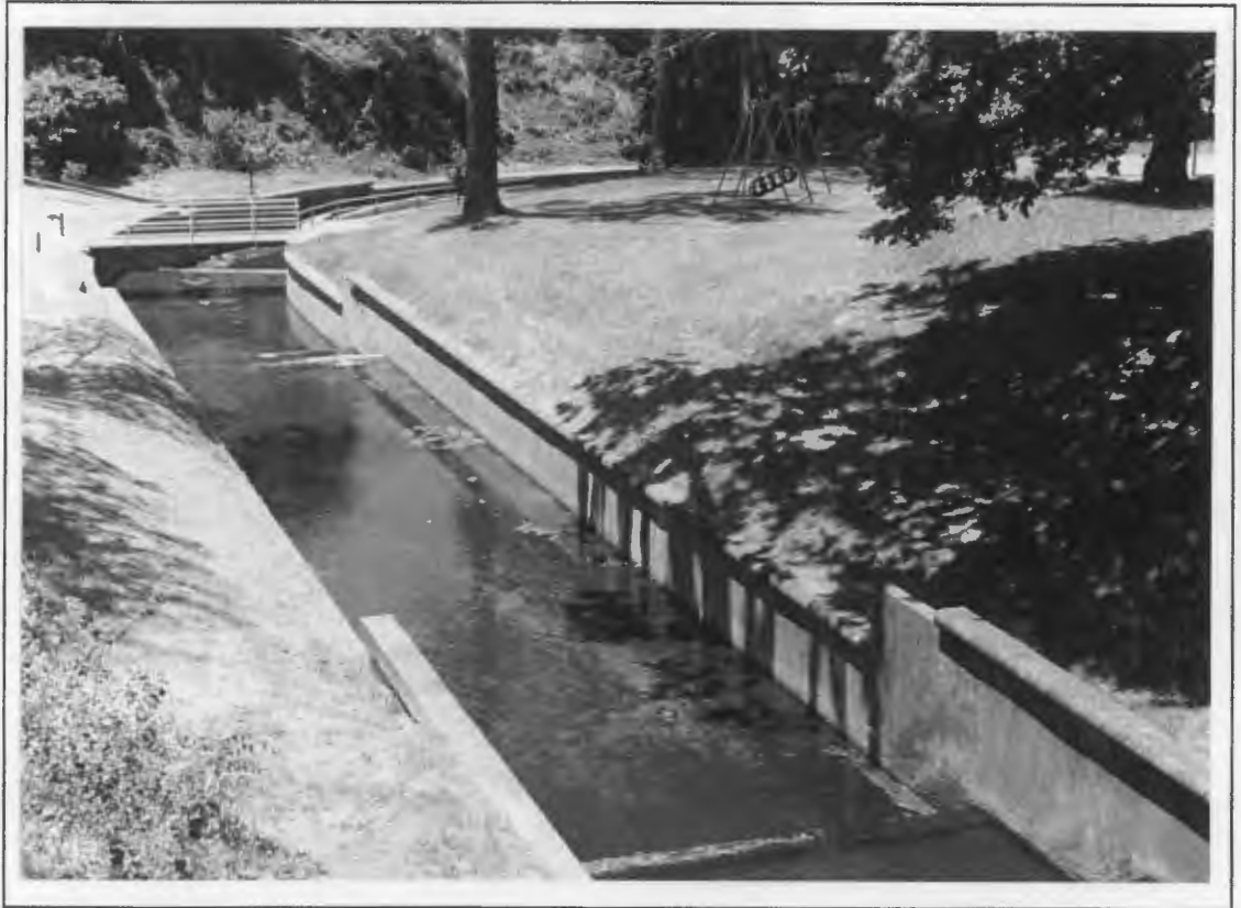
Figure 8.3: A typical section of concrete-lined channel in the middle reaches of the Liesbeek River
