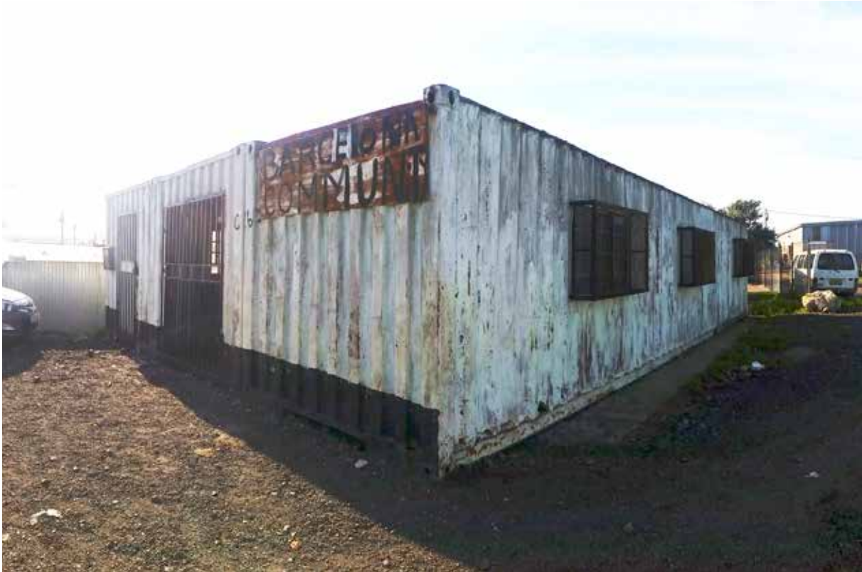
1 Corroded condition of the container hall
