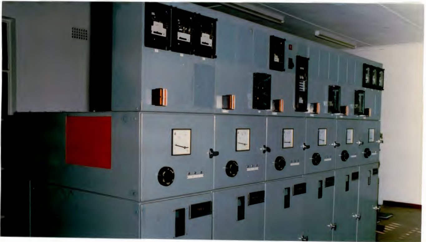
SWITCHGEAR OF BURGER SUBSTATION
