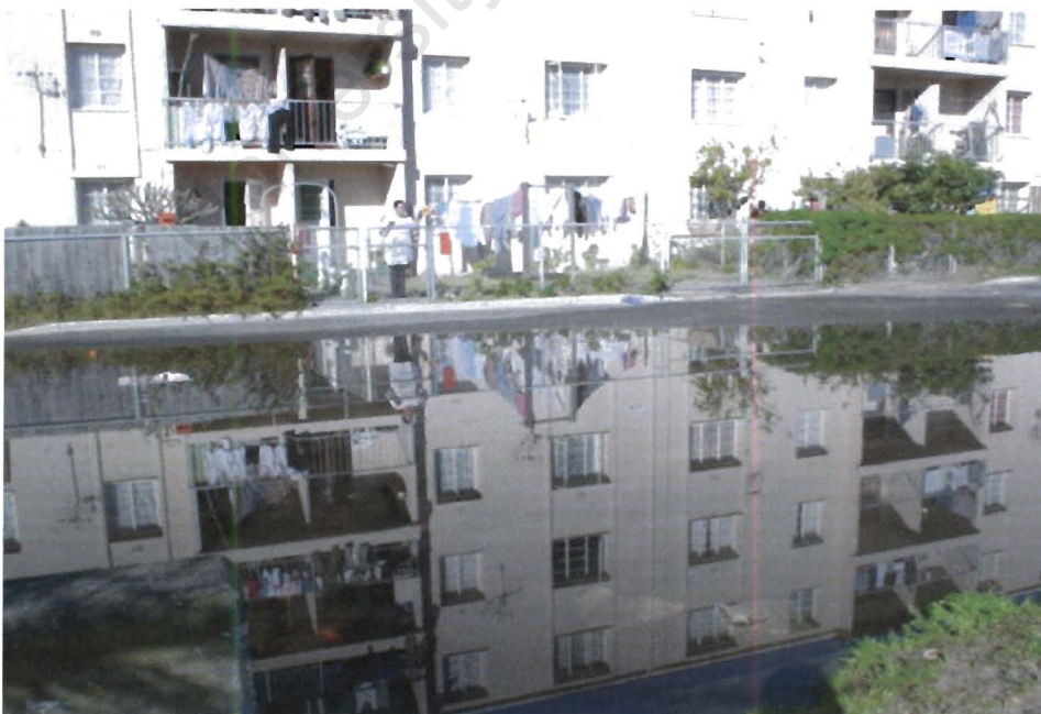
Photograph 18: Blocked and non-existent stormwater drains
