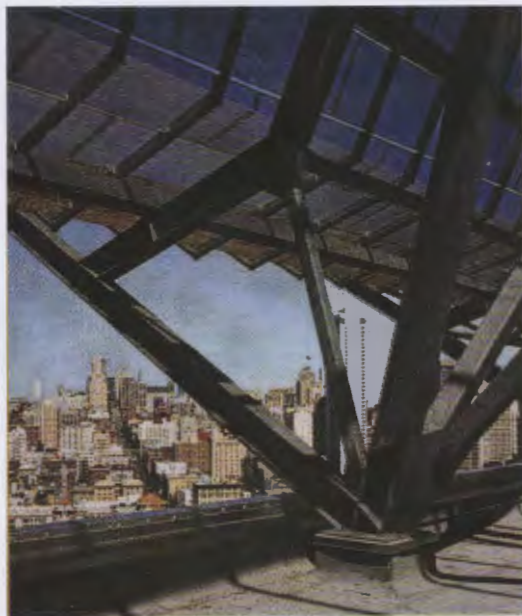
FIGURE 8 _ picture taken from the roof garden on the top floor of the San Francisco Federal, showing the connection of the metal scrim skin
