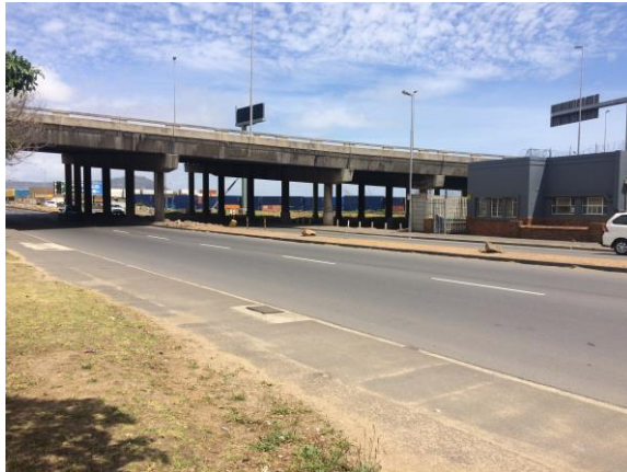
[10] Highway condition of inactive undesirability
