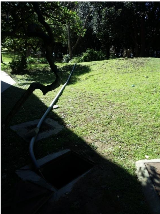
Figure 3-9: Insulated pipe from drain to LMH digester
