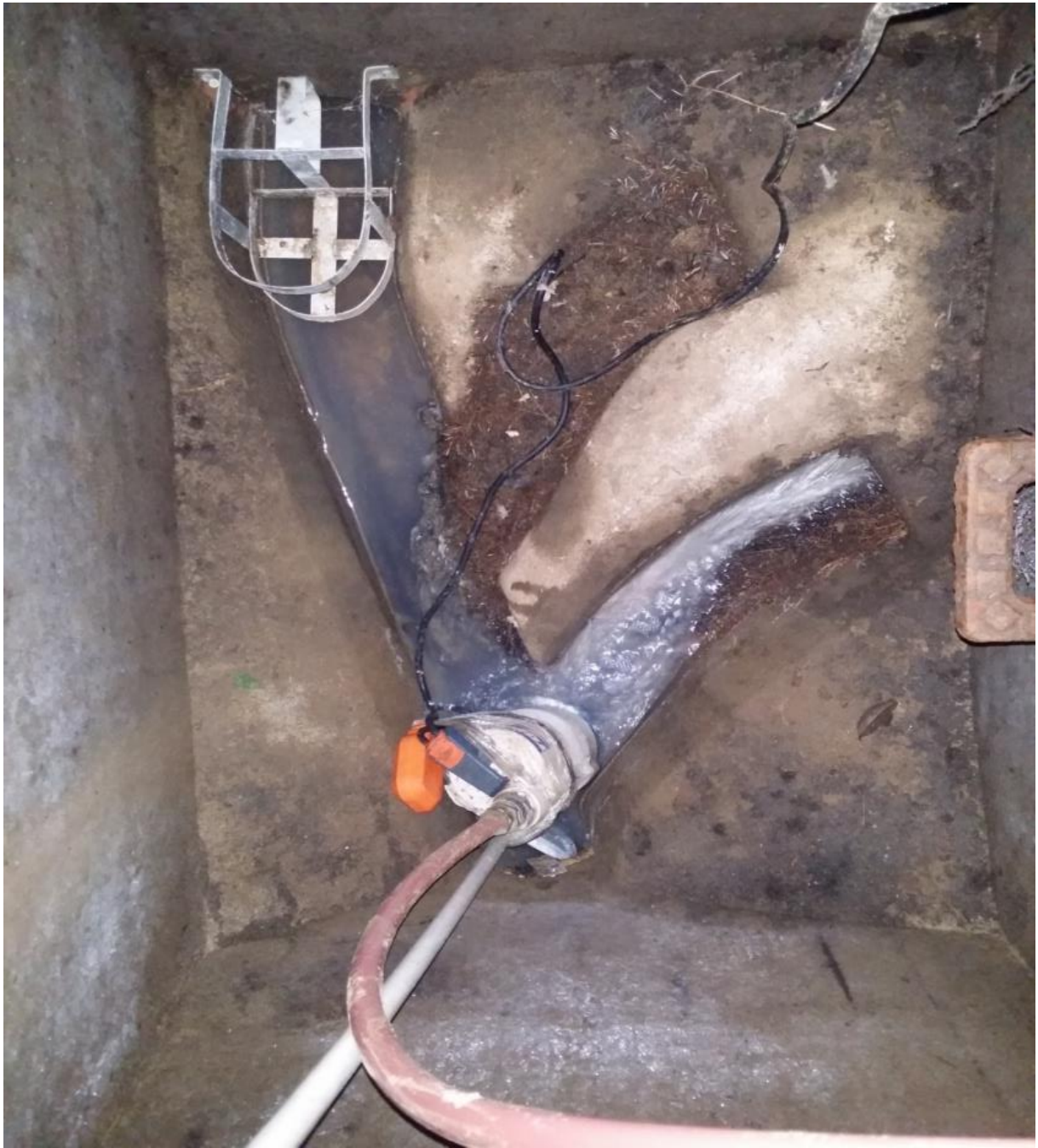
Figure 3-7: Operating submersible pump
