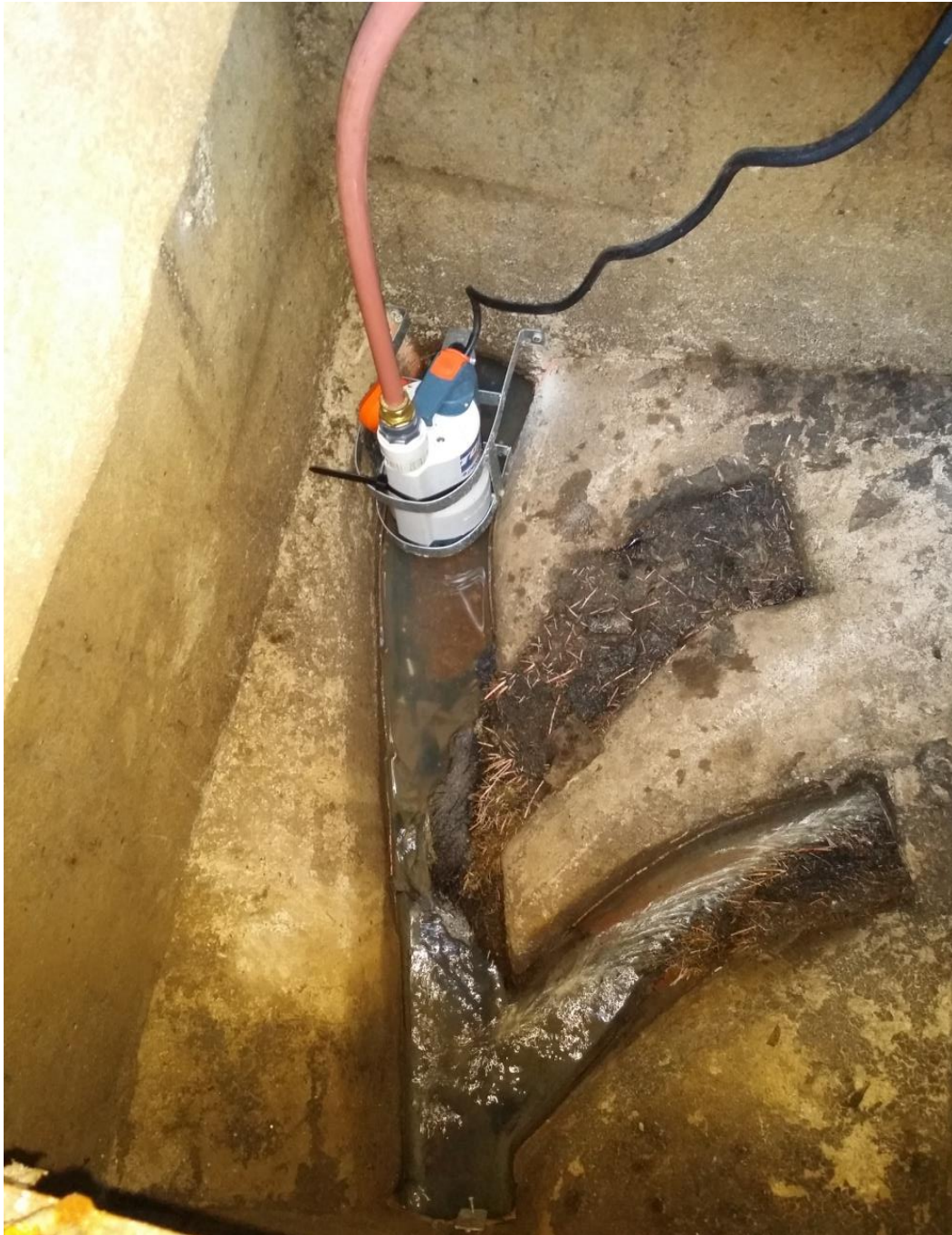
Figure 3-6: Installed submersible pump in LMH residence waste water outlet drain
