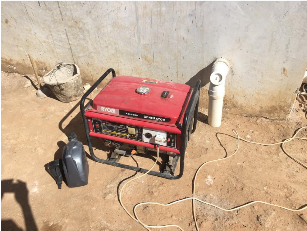
Figure 17: Diesel generator in use behind the main house Source: Primary Survey, Author, 2020
