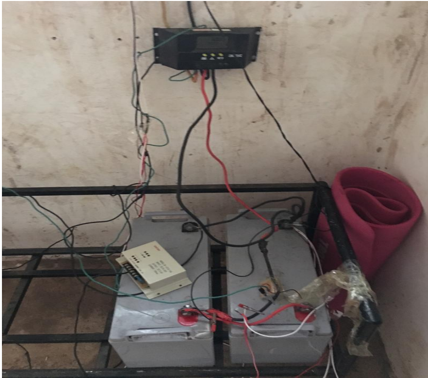
Figure 14: Isaac's car batteries connected and linked to electrical appliances. Source: Primary Survey, Author, 2020
