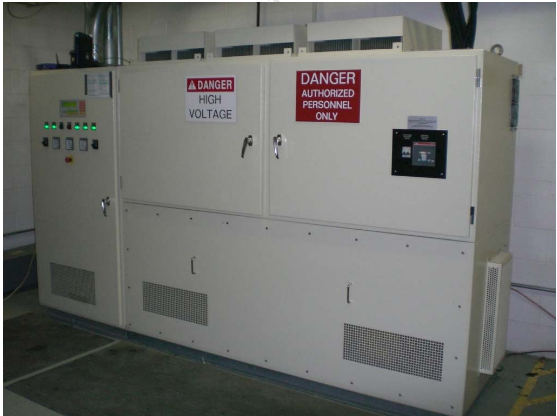
Photograph of the Hybrid Inverter installed in Idaho, U.S.A
