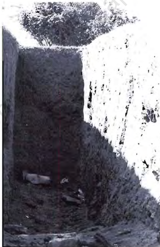
Figure 3.03 : Danielskuil – Building the french drain (Photo by R. Rossouw, courtesy A. Gous)
