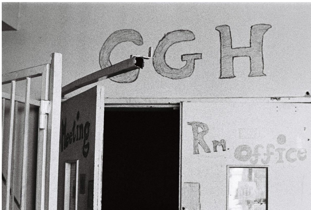
PICTURE 4 - Unhinged gate of the Meeting Room after the brutal police raid of the 31st of January 2022. Source: Tommaso Cosentino
