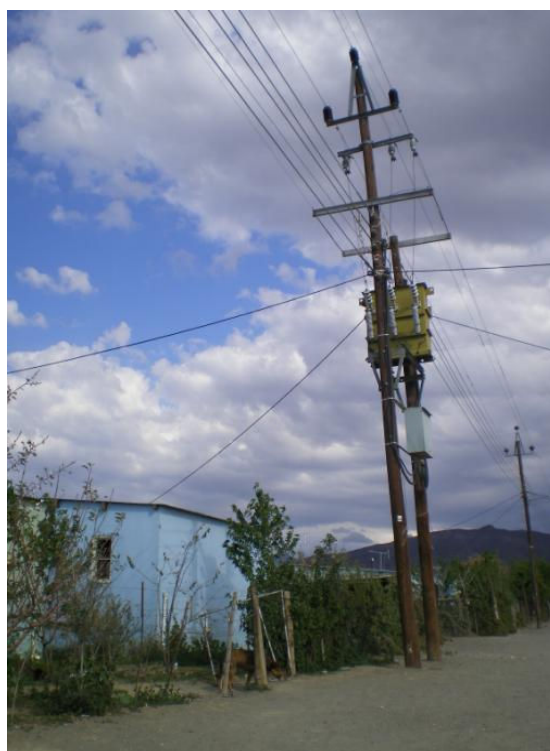
Figure 7: Power lines between houses in the low-income area of Prince Albert
