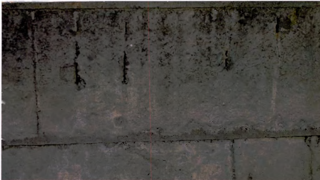
Figure 6.3: Damage caused by carbonation-induced corrosion, Parapet walls 1, Sports Centre Building, UCT
