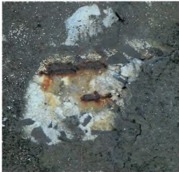
Figure 6.18: Spalling and cracking of concrete due to carbonation-induced corrosion on parapet walls at the Menzies site.
