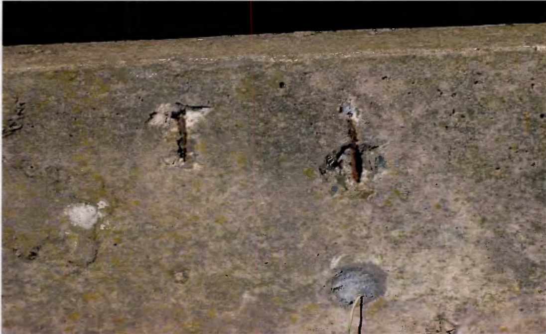
Figure 6.8: Damage caused by carbonation-induced corrosion, 2 nd Parapet wall, Sports Centre Building, UCT
