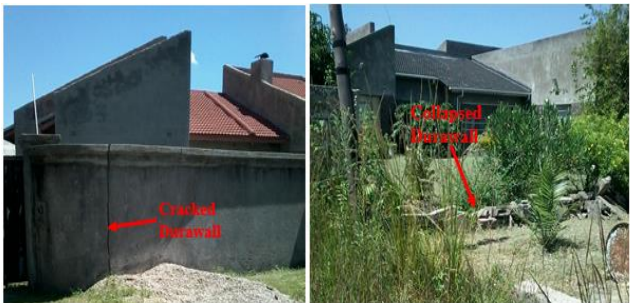
Figure 4.3: Cracking houses built on the Marlborough wetland.
