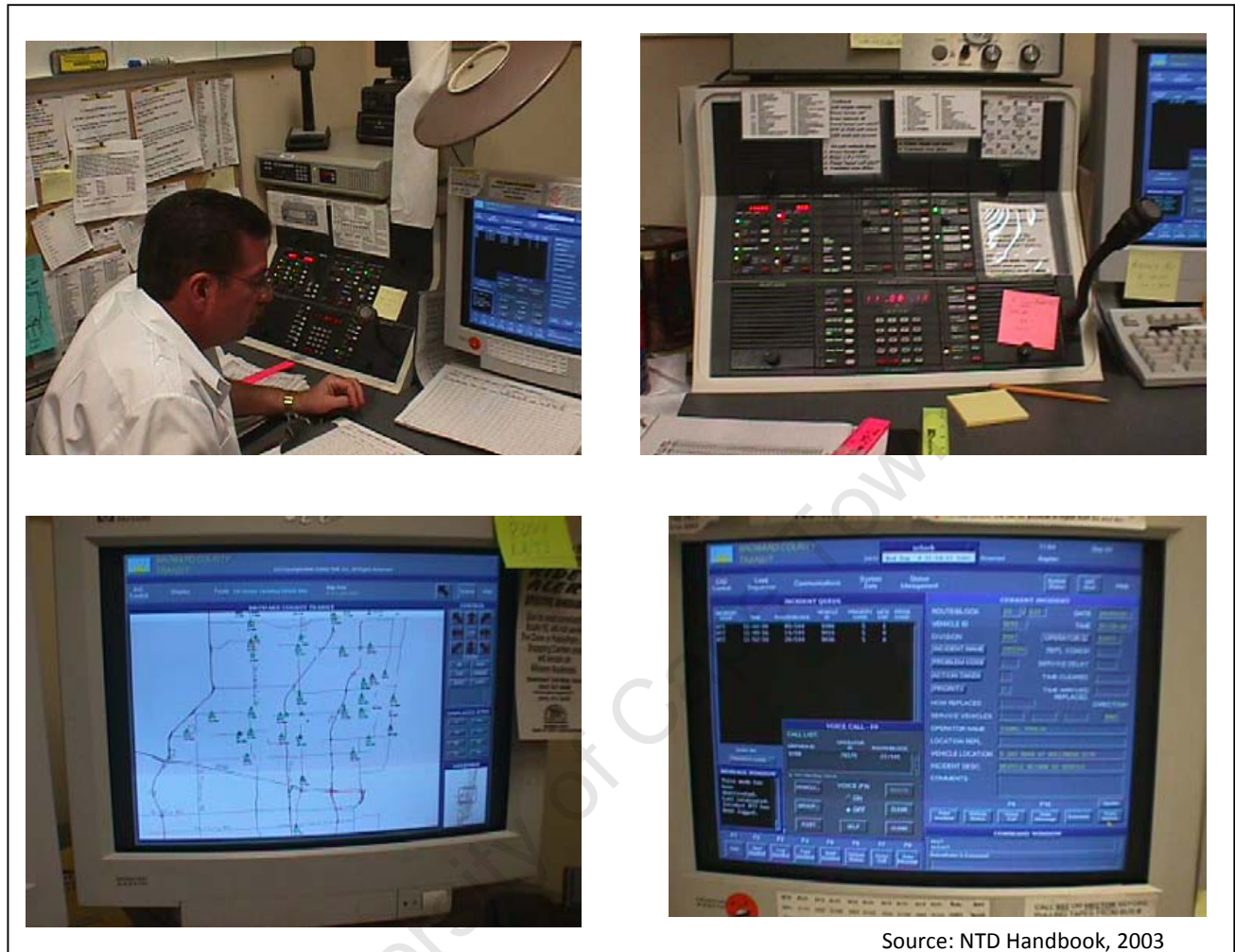
Figure 2.2: AVL control room
