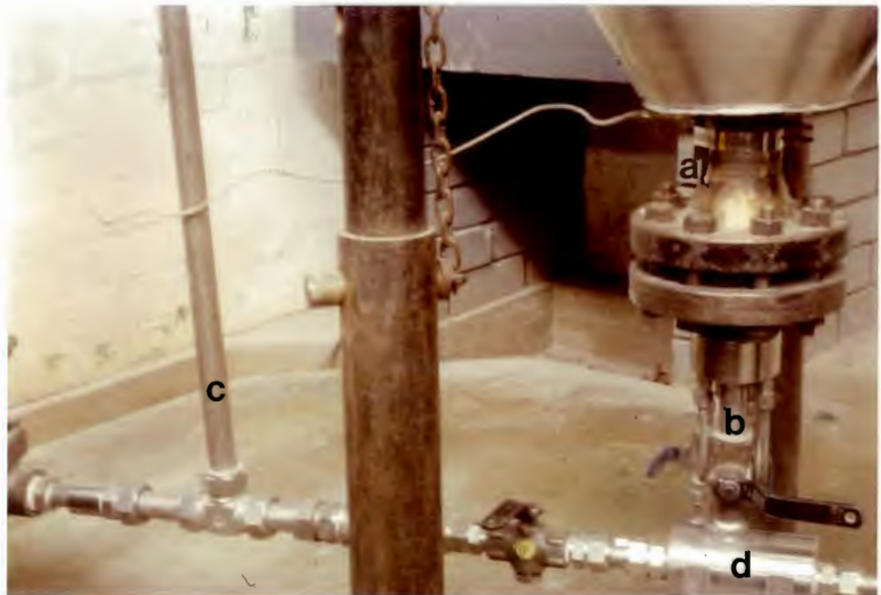
FIG: 3.15 Hopper base assembly showing outside thermocouple attachment (a), ash feed valve (b), prototype air inlet line (c), and venturi chamber (d).
