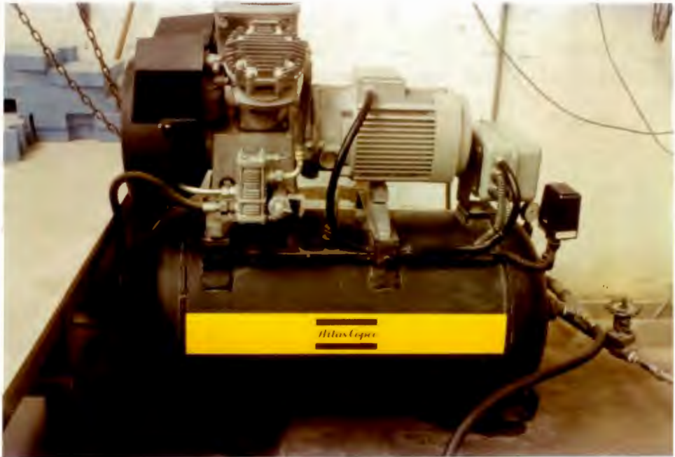
FIG. 3.3: 2.5 MPa working pressure air source with attached 350 l receiver.
