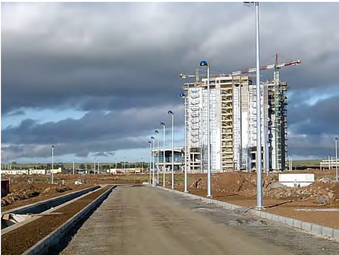
Photo 2: Construction of B05 in parallel with infrastructure and civil works for the precinct in 2002
